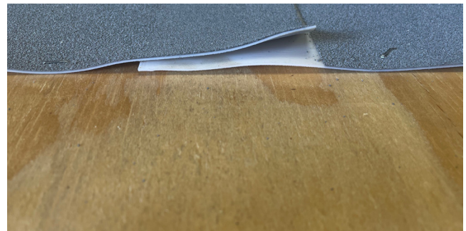
SEAM REQUIRING REPAIR: REPAIR PER ABOVE STEPS
